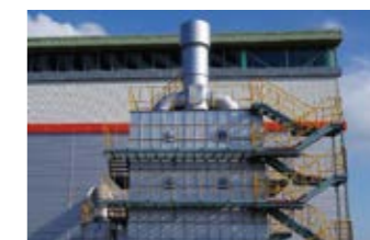
Exhaust gas treatment system
